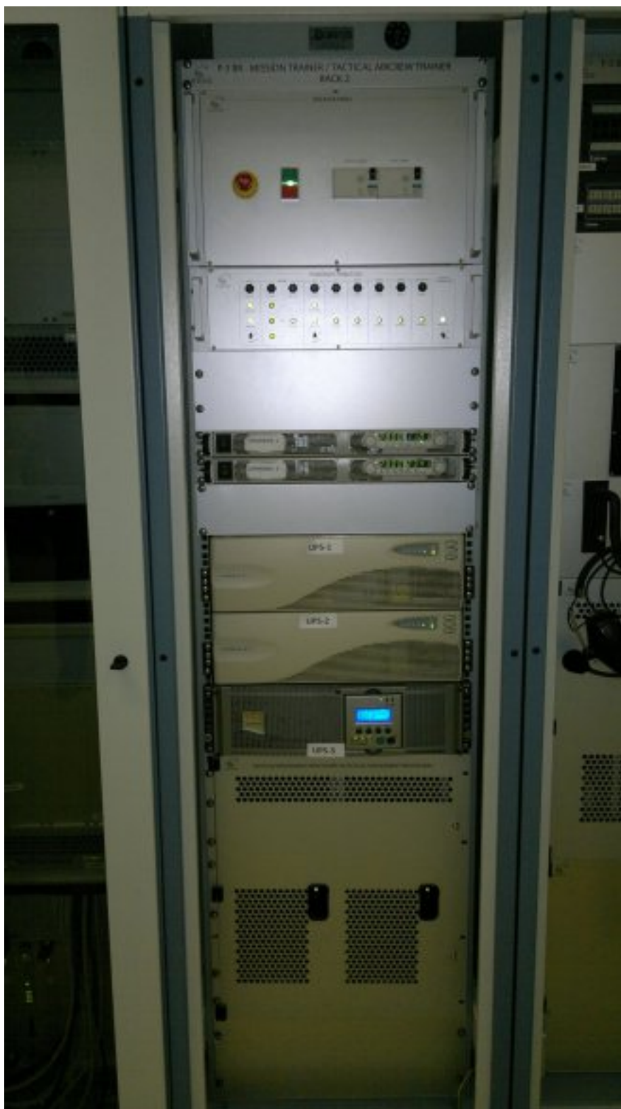
Figura 7 – Breaker Panel, Power Distribution, TMP#1 e TMP#2
