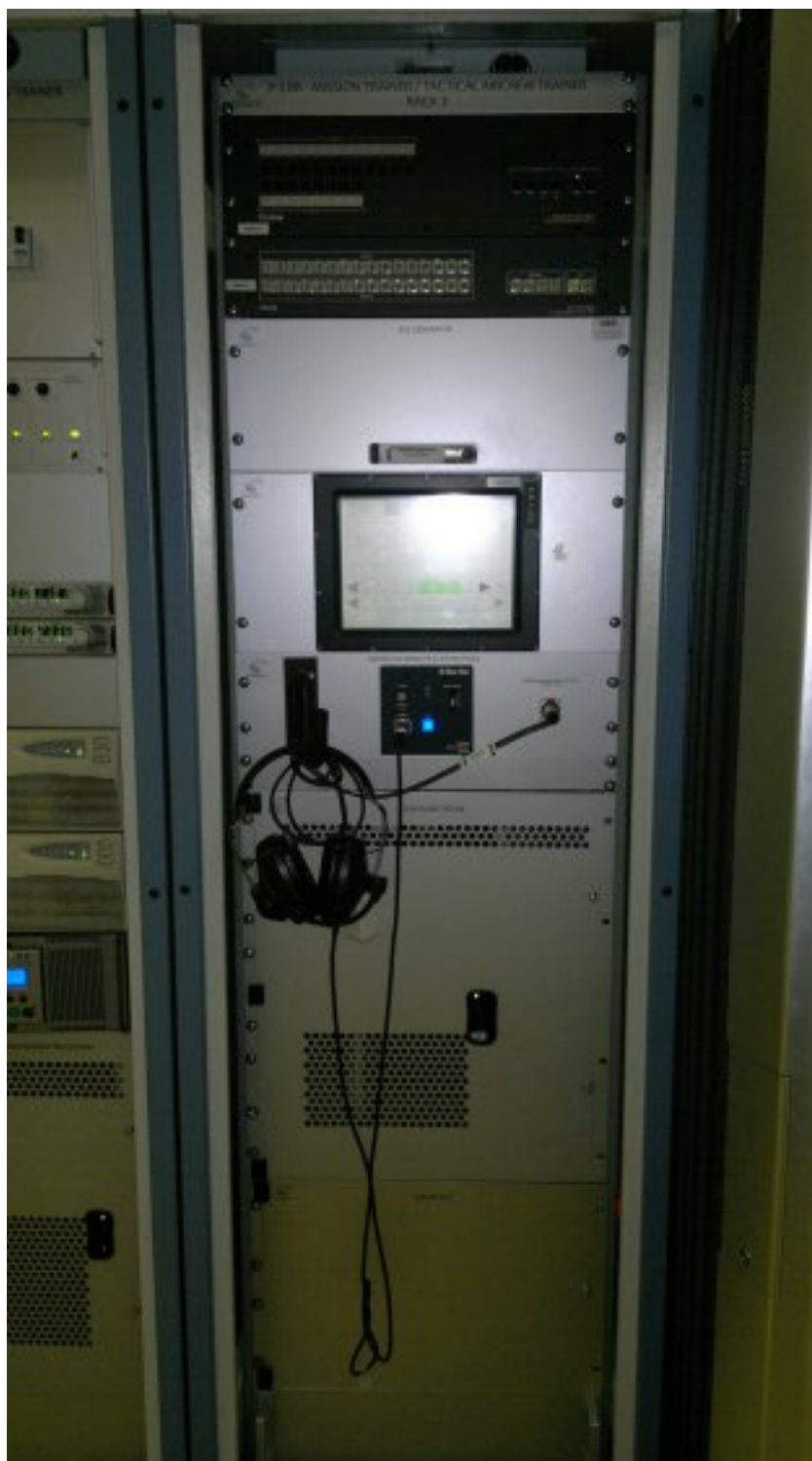
Figura 6 – Sistema ESS Generator, ESM Workstation e RADAR EDM
