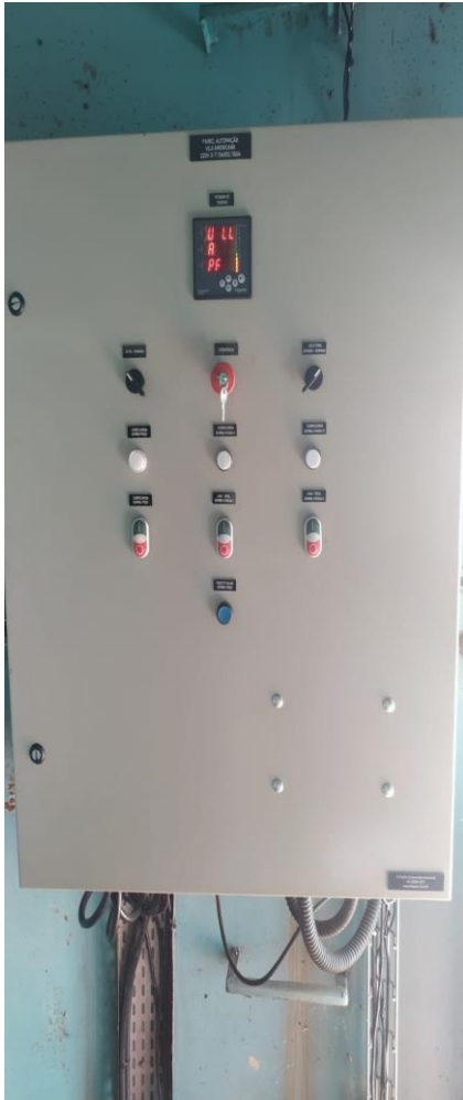
Foto 19 – Frontal do Painel bombas
