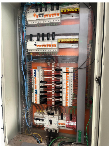
Foto 5 – Interior QGBT Rancho Cmdo 4ªRM
